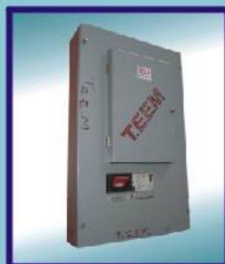
E02 Main Switch
